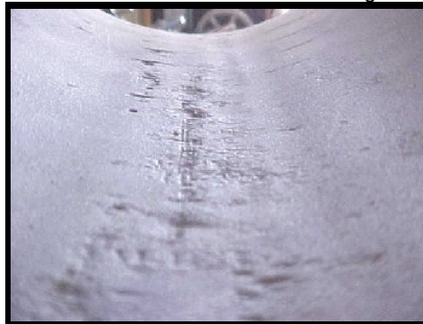
This shows all the DAMAGE caused by the application to the inside of the Heat Exchanger Unit
