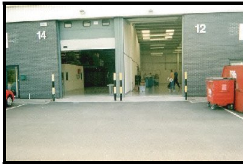
Front view of two warehouses and production areas needed to be re-coated.
