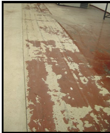
The damaged area is shown above with the existing coating being removed
