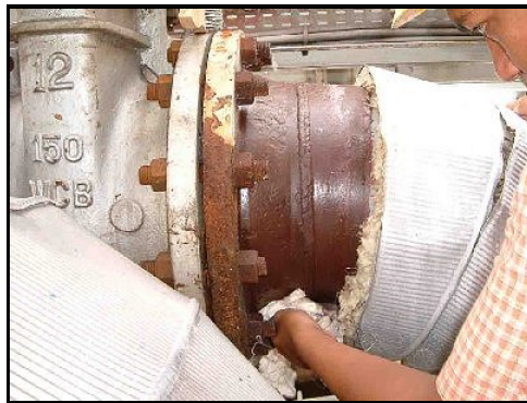
Part of the pipe system needing repair.
